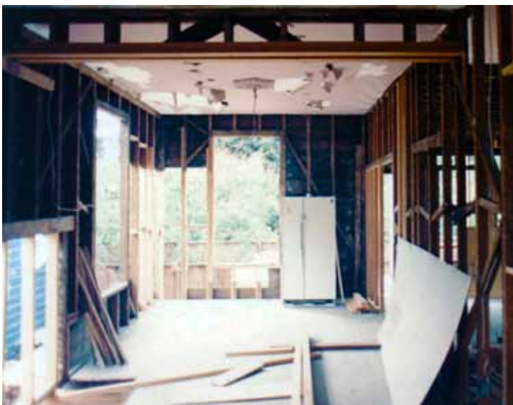
Looking toward the original dining room from the parlor, this image shows stripped walls and new framing. An original ceiling medallion and remnants of pocket door framing were exposed when the lowered ceiling was removed.
