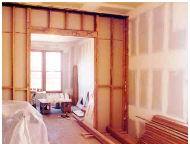
Looking toward the front parlor from the dining room, this image shows new pocket door wall under construction, new double windows in front, and new sheet rock.
