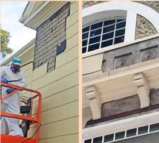
Top: The house shown with various modern alterations and missing ornamentation and brackets. Bottom left: Siding being removed to show two patterns of wood shingles remain underneath. Bottom right: Intricate details also were found below the attic window. Image: homeowners.
