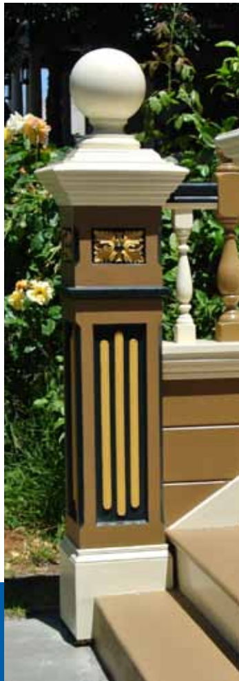
New stair railings and balustrades were constructed with intricate details showcased by an attractive color scheme.
