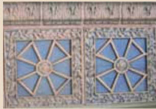
For the façade restoration the Fong family made sure the beautiful historic tile was maintained.
