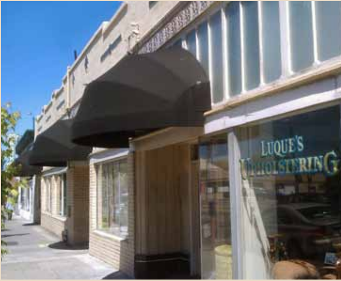
Some of the Powell Building's details had been obscured by the addition of large bulbous awnings.
