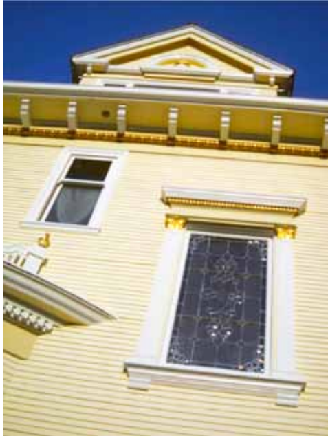
Details on the exterior. This view shows the upper stairwell window with Corinthian pilasters; the bay-window cornice with dentils and urn finial; and the roof eave with modillion brackets. Photo: Woody Minor.
